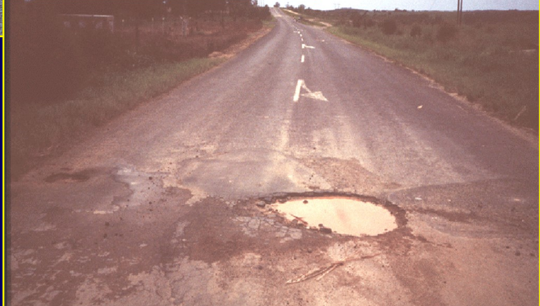
POTHOLES : Water & Loads ...
